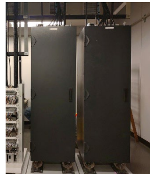
CBTC wayside equipment
